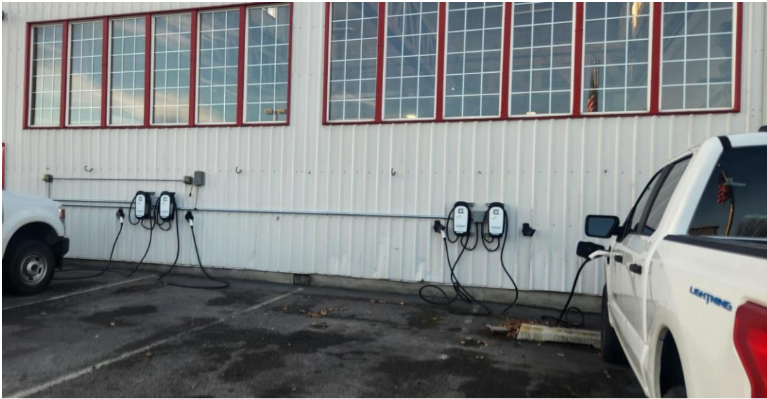
Figure 10: Make-Ready fleet charging installation at City of Spokane Park Operations.
