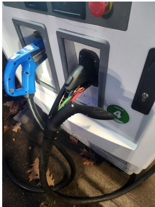
Figure 14: Connector cable damage identified during an inspection.
