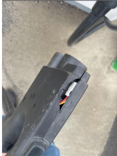
Figure 15: DCFC connector cable latch missing
