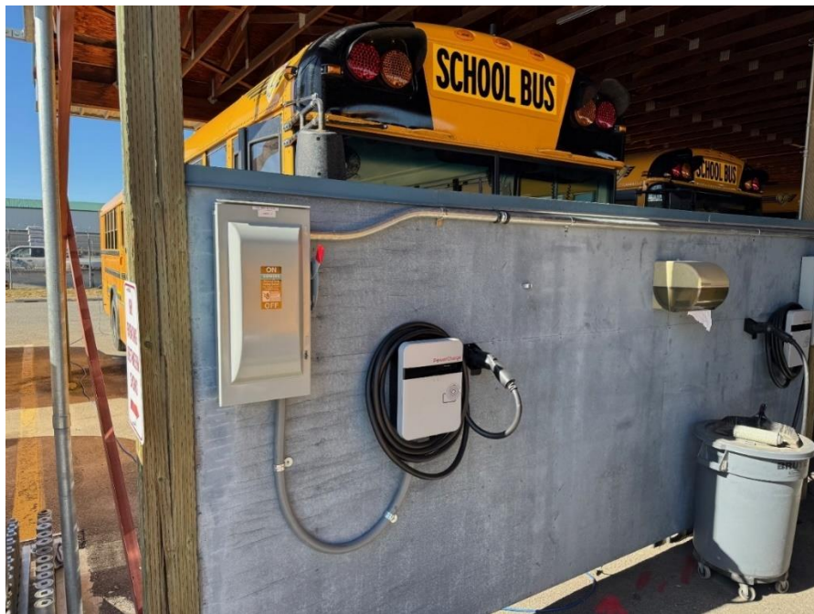
Figure 23: West Valley SD Charging installation.
