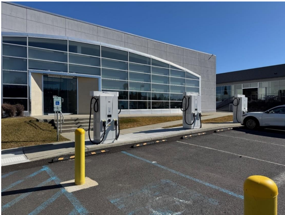
Figure 13: Wendle Ford DCFC Installation
