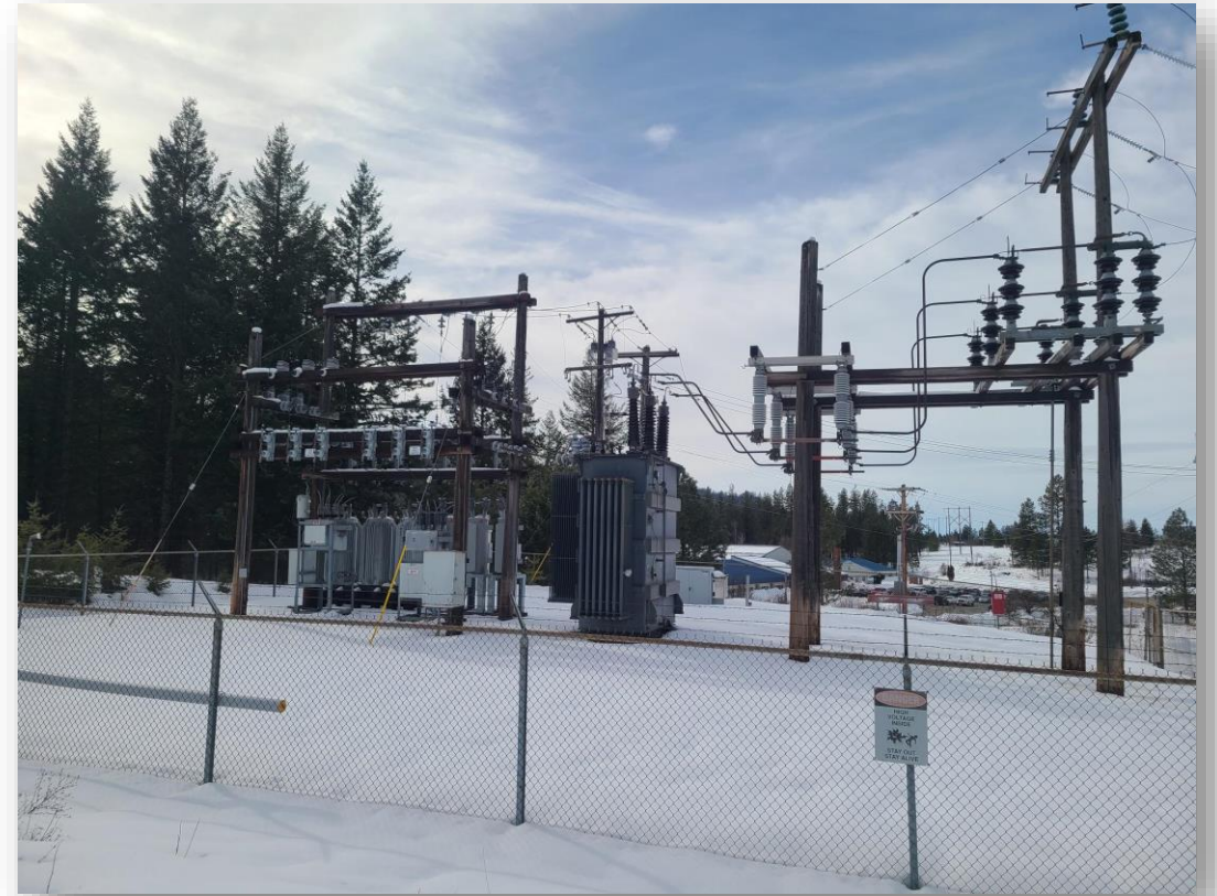
Avista's O'Gara 115kV / 13kV Substation, South of Harrison, ID
