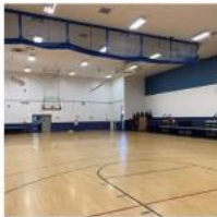
Heating & cooling area
