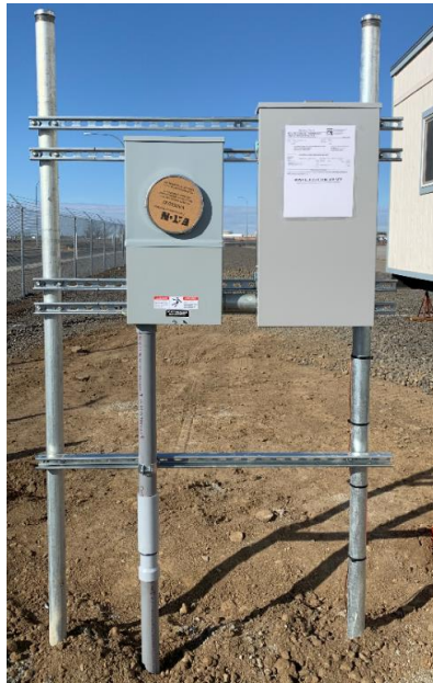
Figure 4.14 – 200A Pipe Meter Pedestal Install Photo
