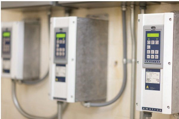
Programmable variable frequency drives (VFDs) control pool pumps more efficiently. The pumps no longer have to run at 100 percent all of the time.
