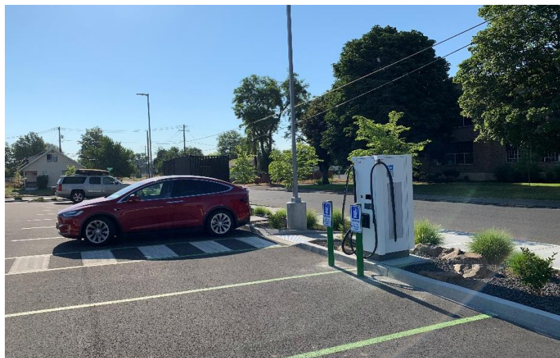
Figure 12: Completed DCFC site at The Hive – Spokane, WA (2022)
