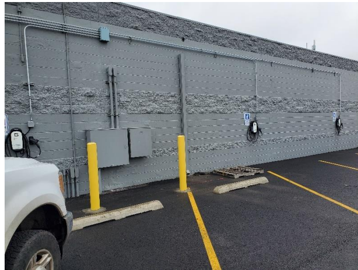
Figure 8: Fleet charging installation
