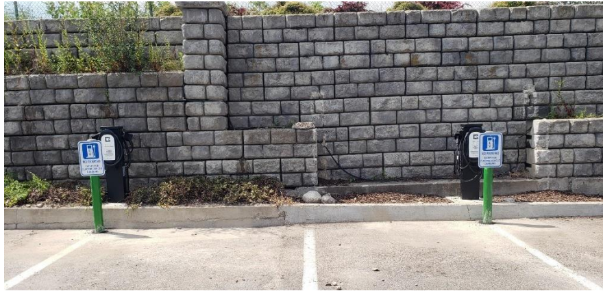
Figure 7: Workplace charging installation
