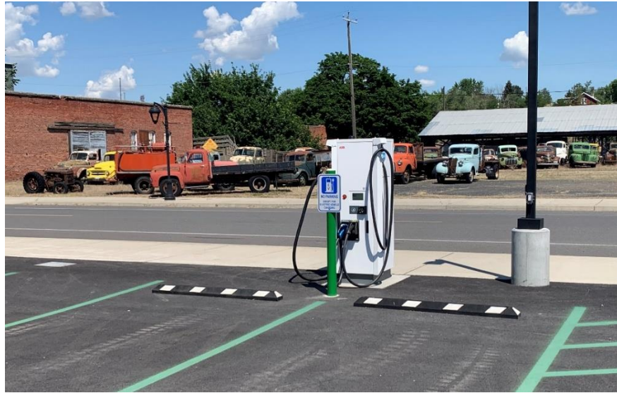
Figure 13: ABB Terra 184 DC Fast charger – Sprague, WA (2022)
