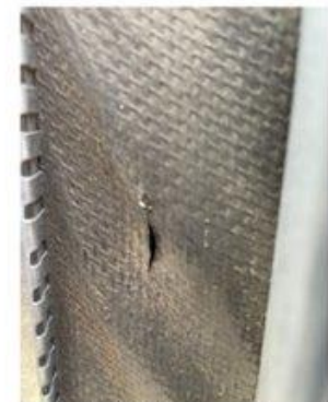
Tear in Fabric Duct Transition
