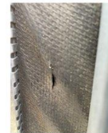
Tear In Fabric Duct Transition
